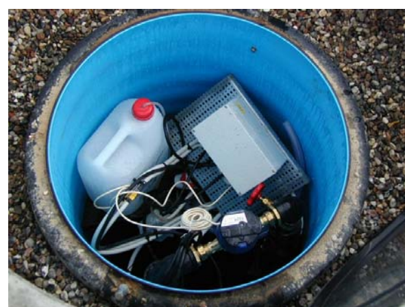
Figure 3 Leachate collection and pumping well.
