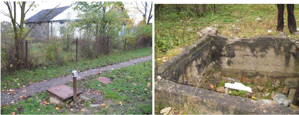
Figure 12. Drinking water borehole in Bolshiye Polja (left); Abandoned rural well (right)
